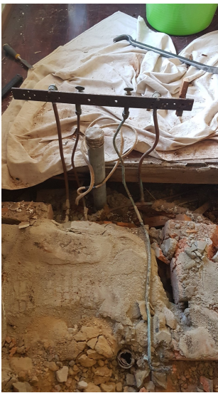
Termite-damaged flooring removed around access and threshold areas.
