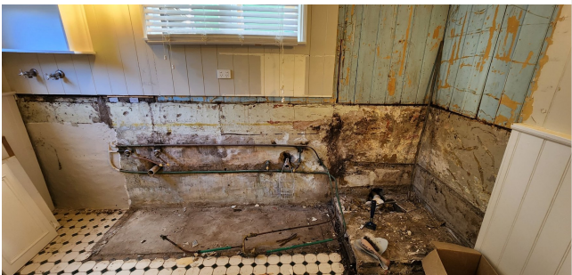
Bathroom/wet-area damage exposed after removal of fixtures and linings.
