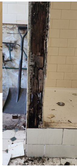
Concealed timber damage beside wet-area wall and shower zone.
