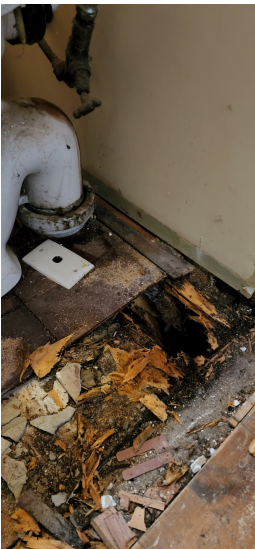
Rot and floor deterioration around wet-area plumbing.
