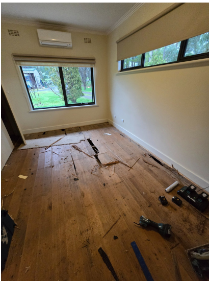
Visible room works became a concealed subfloor issue once material was removed.
