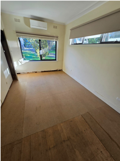
Rotten and failed timber removed from affected areas.
