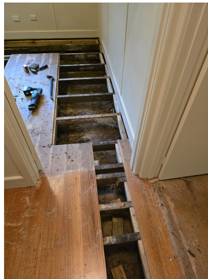
Floor sections were opened to expose the true condition of the subfloor and framing.
